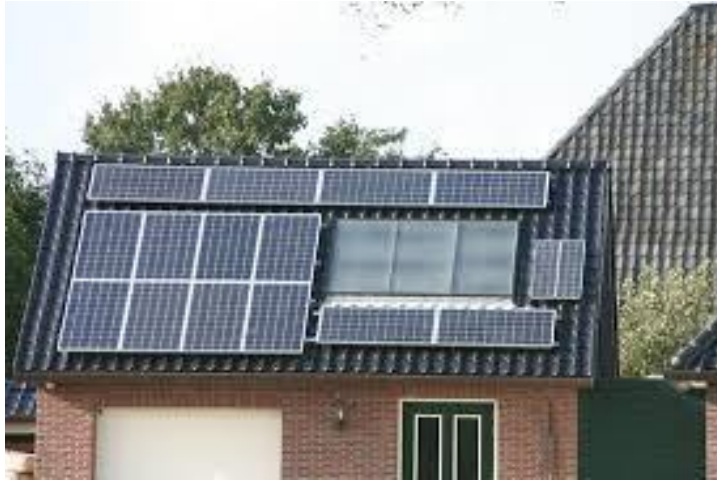
From BAPV on Buildings
