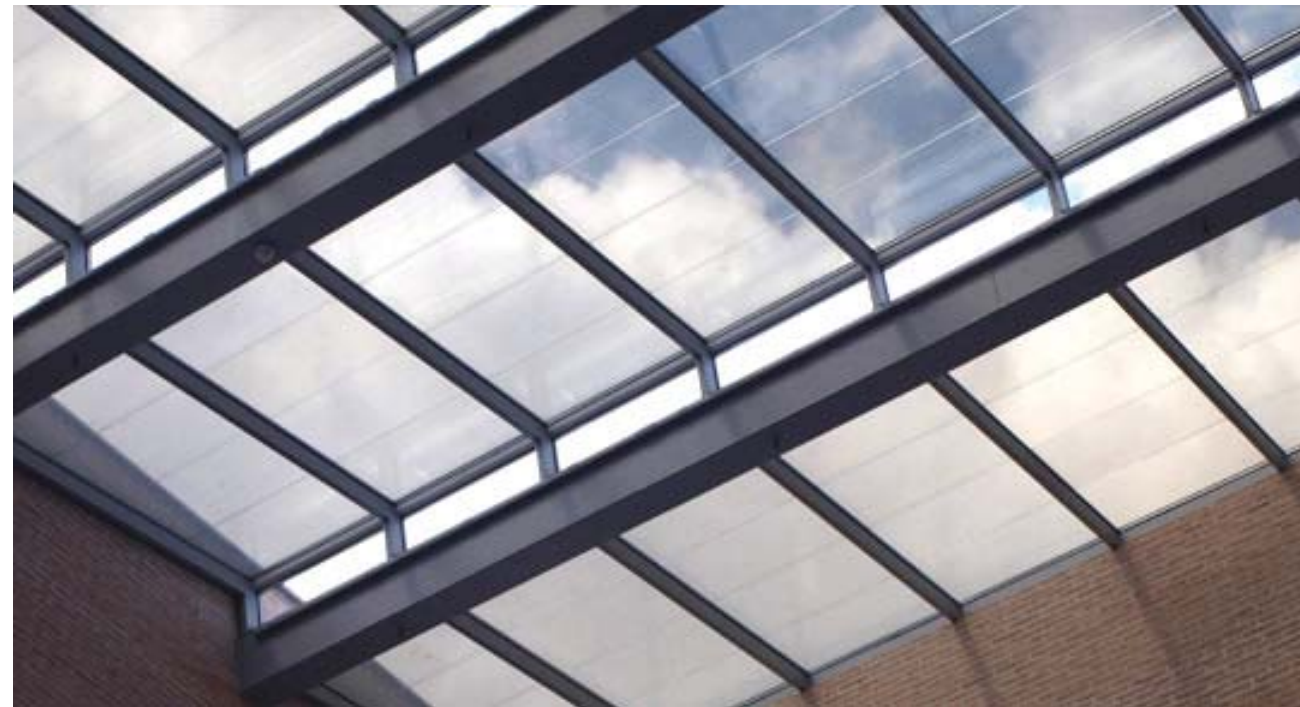
Onyx Solar Photovoltaics Transparent Glass installed into San Anton Market, Madrid (Spain)
