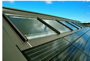
Smart grids and net zero energy buildings
