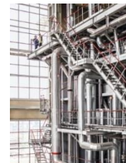
Process Industries and Drives
